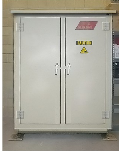
EXAMPLE 5F: Hazardous Materials Storage Container/Cabinet
